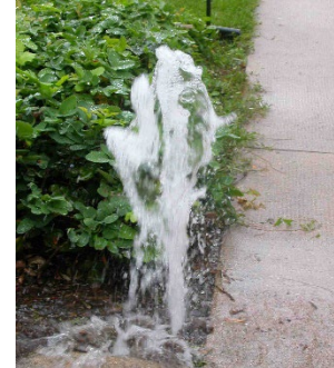
Runoff and soil erosion caused by broken irrigation equipment
